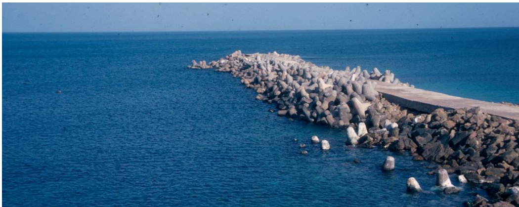
Figure 2 Damaged tetrapod breakwater in El Kala, Algeria.
