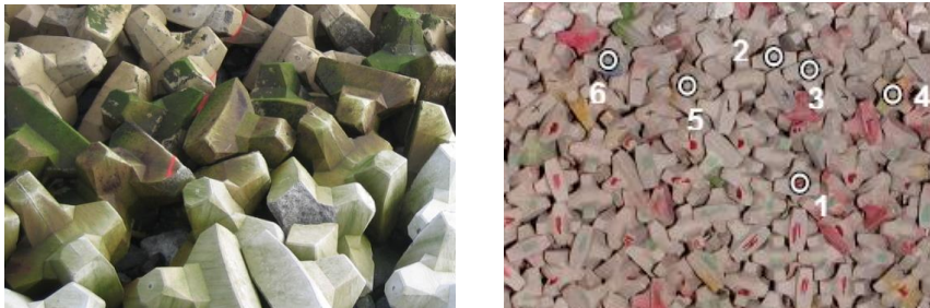
Figure 4 Broken units in the prototype (left) and rocking units registered in model tests (right). Revetment with Accropode™ I (6.3 m 3 ).
