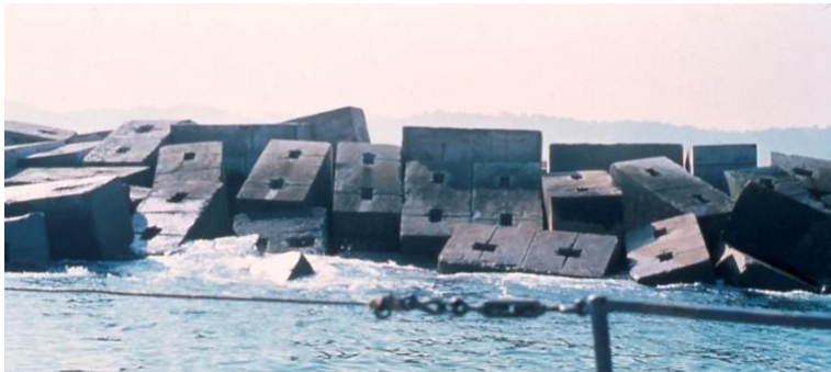
Figure 1 Example of breakwater armoured with large rectangular blocks (Port of Algiers, Algeria).
