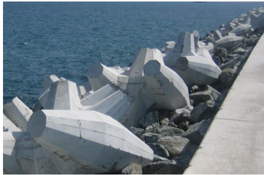
Figure 6 Example of damaged Core Loc™ Breakwater where the whole armour layer settled due to compaction and sliding on the rock underlayer.
