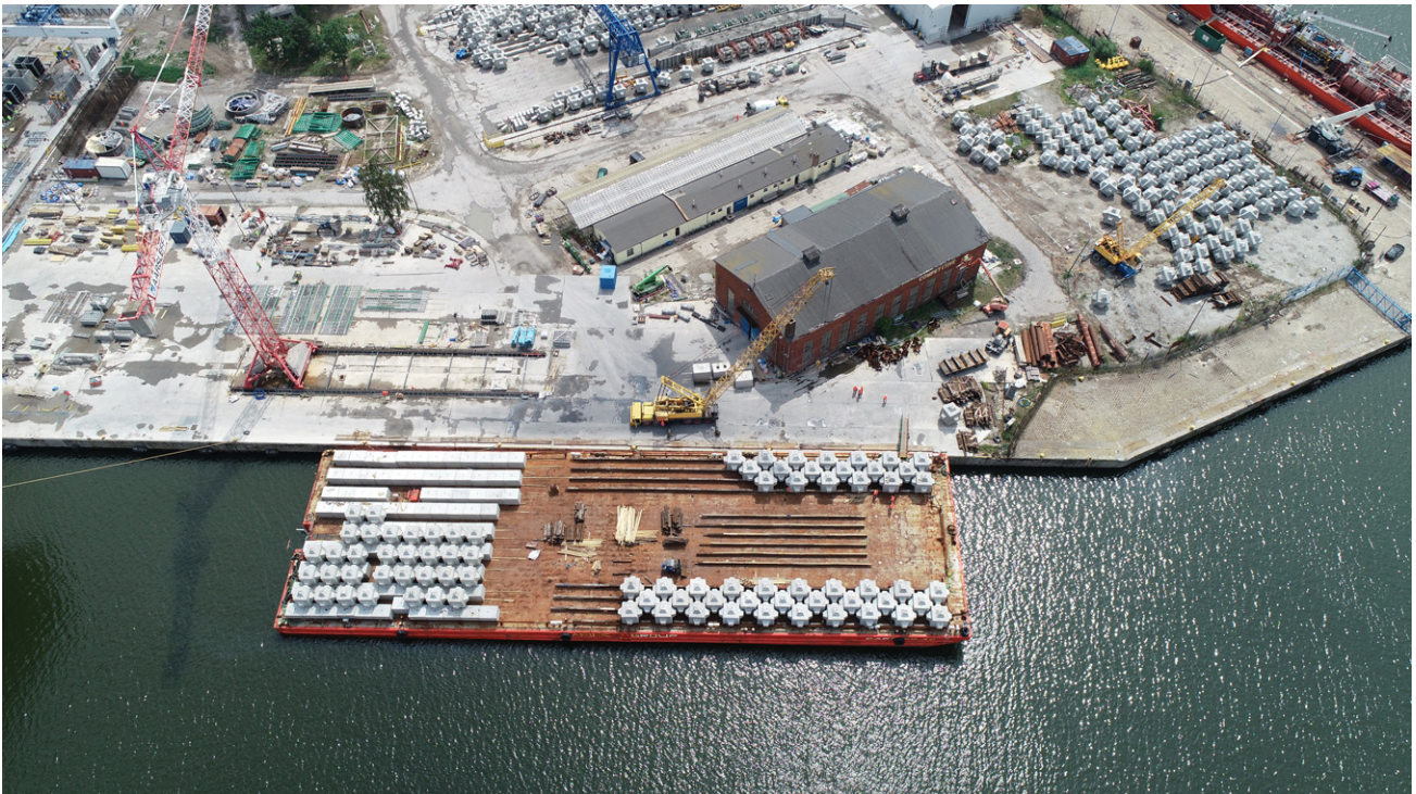
Figure 14. Production and barge placement of Cubipod at Aarsleff Biz in Świnoujście, Poland
